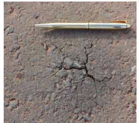
Figure 1 – popping in pavement surface
