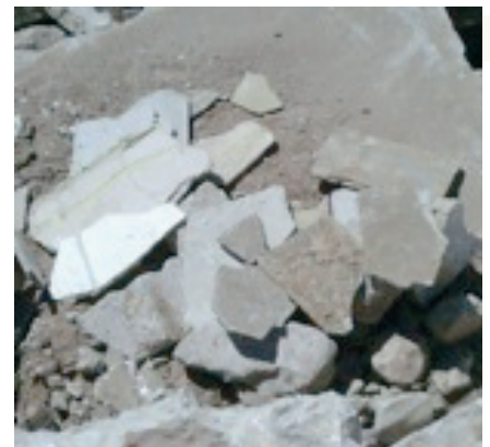
Figure 1. Asbestos sheeting in demolition concrete (rejected at receiving point)
